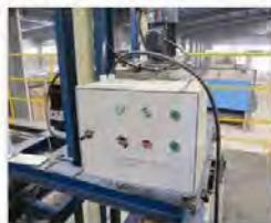
液压站配电箱 Hydraulic station distribution box
