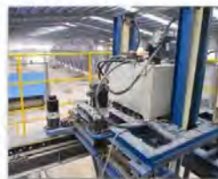
液压泵站 Hydraulic pump station
