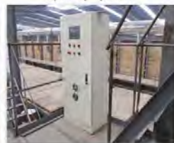
编程控制柜 Programming control cabinet
